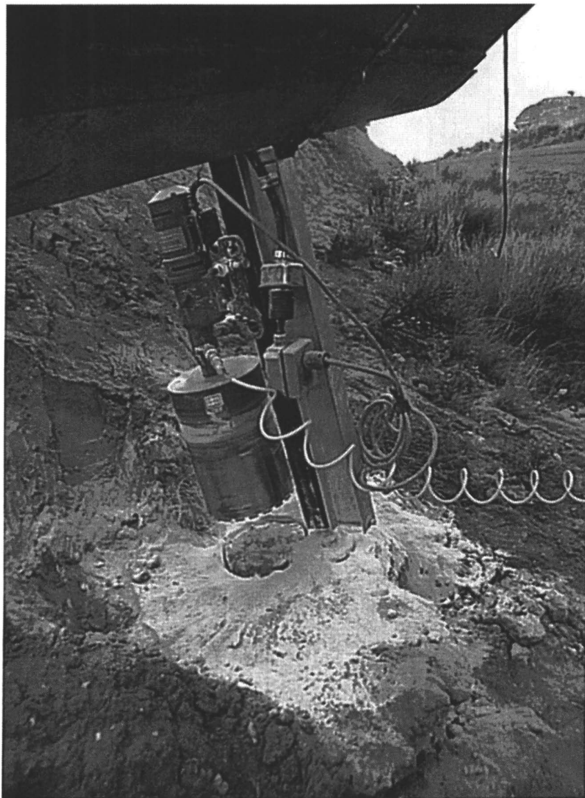
Figure 1. Air-rotary coring apparatus for obtaining intact cores of the Plio-Pleistocene Unit, White Bluffs, Hanford Reservation. Diamond-bit core barrel (10-inch diameter) was attached to a track-mounted hydraulic motor. The entire apparatus was affixed to a backhoe bucket in order to obtain cores at any angle.
